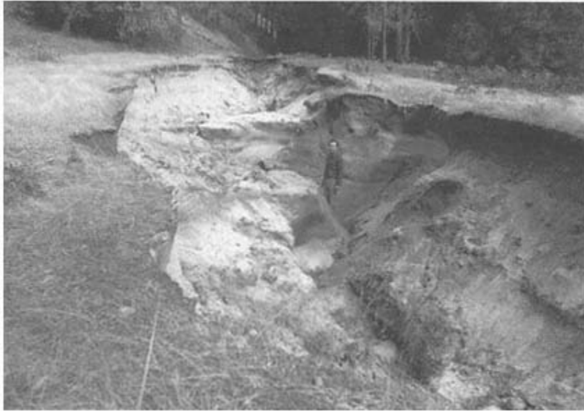
Gullying is unmitigated waste. Loss of highly erodible soil in the Trinity River watershed destroys usable land and chokes salmon spawning habitat with blankets of silt. (Bureau of Reclamation)
