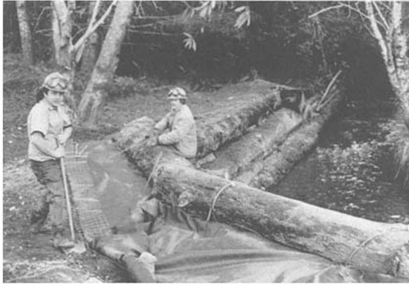
Fixing a stream. California Conservation Corps workers are restoring a streambank of a Mattole River tributary that had been damaged by poor land-use practice. (Alan Lufkin)
