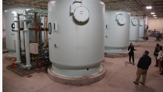
Des Moines Water Works nitrate removal facility. (Kelsey Kremer / The Des Moines Register)
